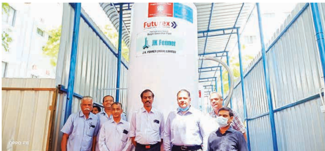
Donation of Oxygen Generating plant in Madurai
